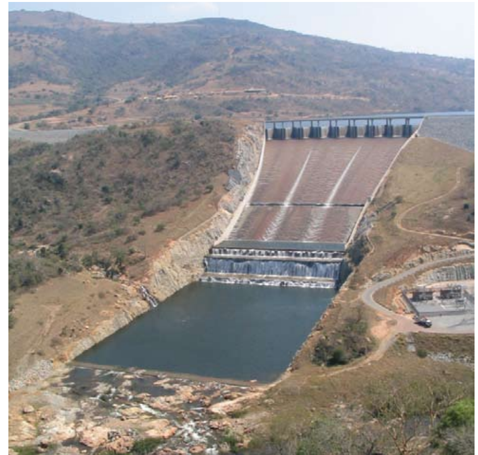
Maguga/Lake Matsamo dam, Swaziland, controlling outflows in the Komati river system / Werner Comrie
